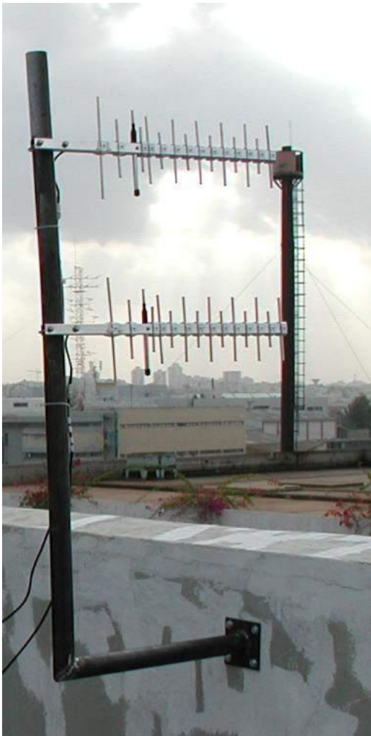
An Example of Correct Installation of Directional Antennas
