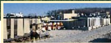
Industrial Battery Plant
